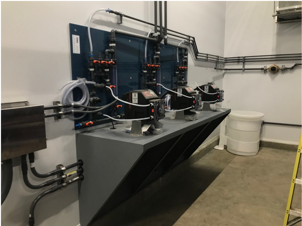
Chemical feed pumps that will provide the necessary chemicals to remove manganese and arsenic.
