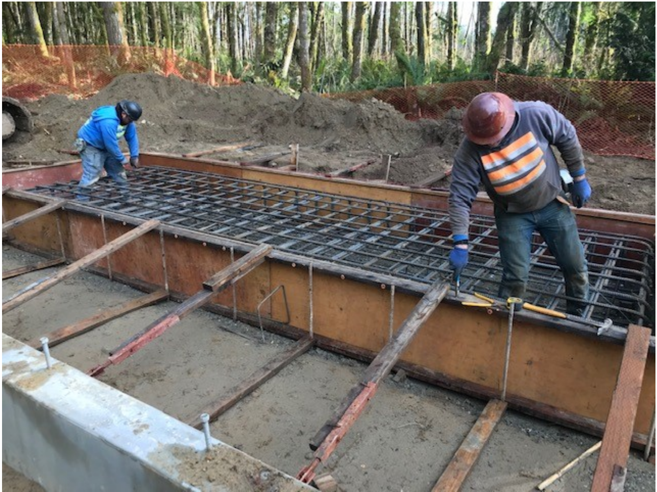
JMG Constructors tying iron rebar together for chlorine contact tank concrete support pad.
